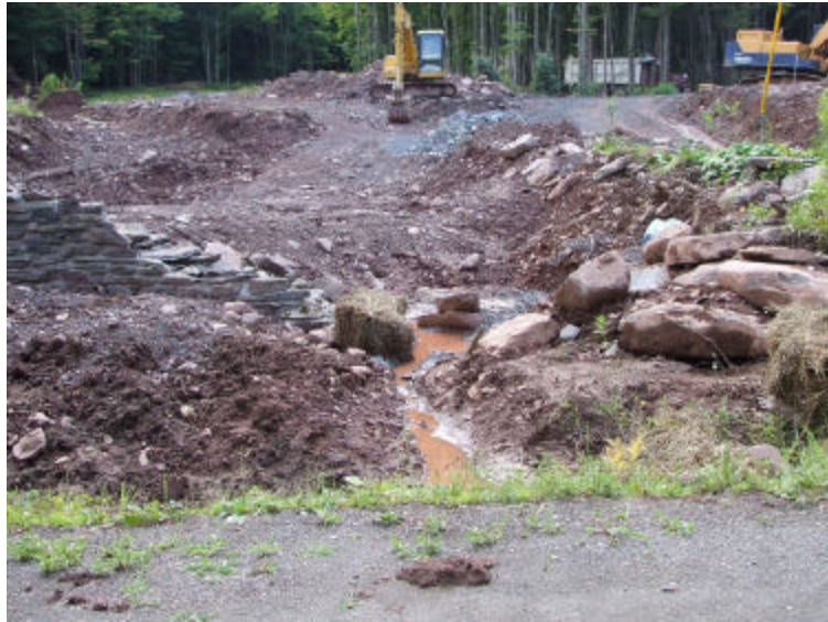
Figure 2.9 Improper sediment controls during construction of a major subdivision
