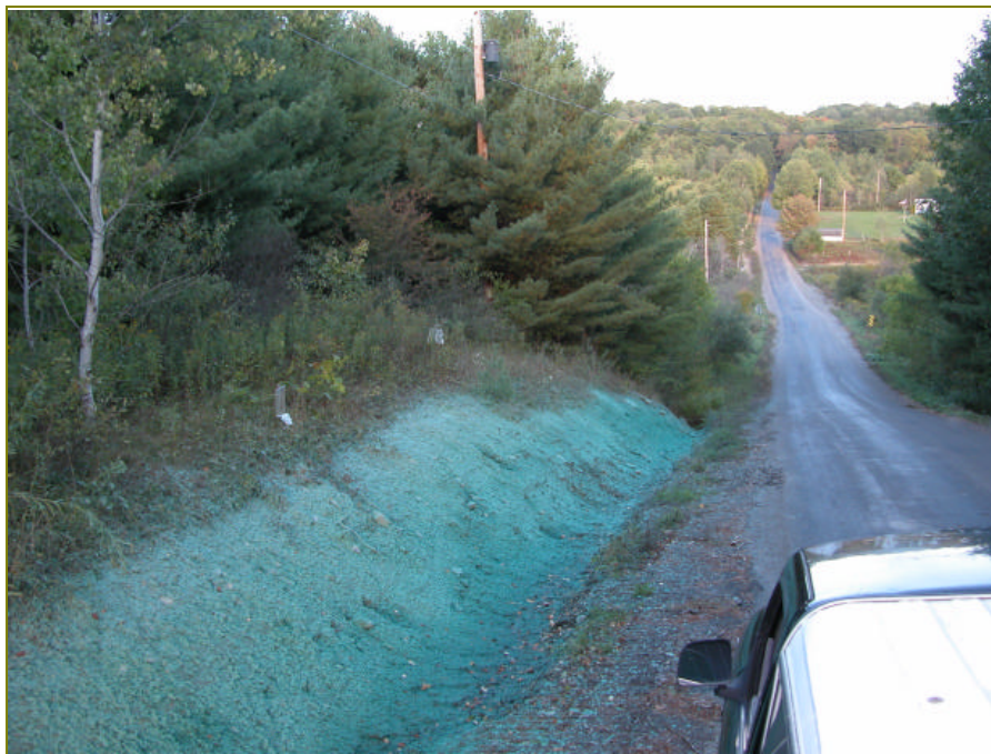
Figure 5.1 Example of a hydroseeded ditch that should be done early in the season to allow sufficient growth.
